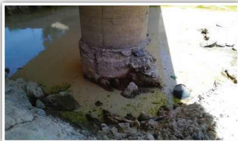
❌ A riverbed with debris and other obstructions
