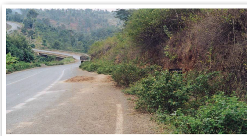
❌ Carriageway obstructed by bushes
