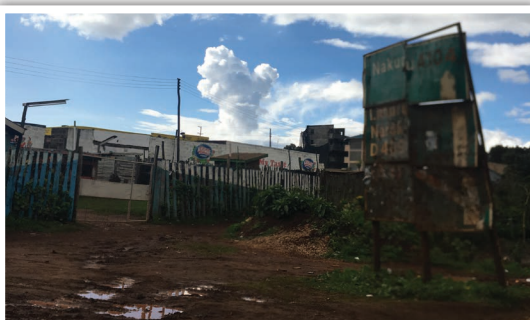
☒ Corrosion of traffic signs
