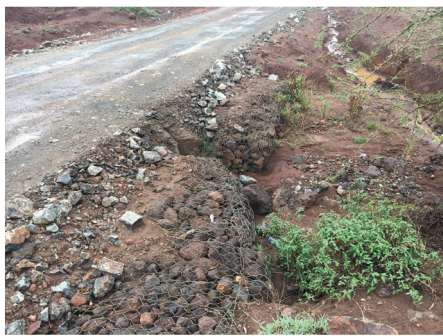
A rough shoulder
