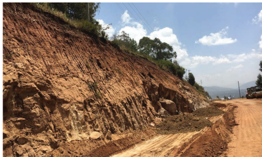
Absence of warning sign
