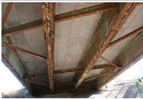
Steel structures deterioration
