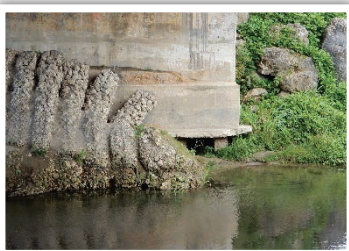
☒ Erosion around bridge abutment
