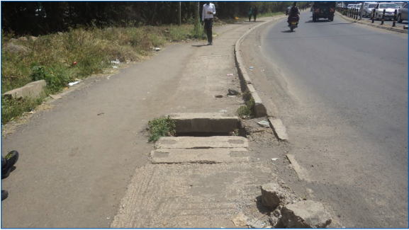
7. Footpath: Openings unsafe for pedestrians
