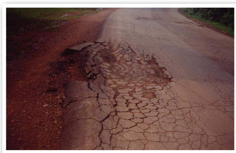
❌ Typical heaving causing depression
