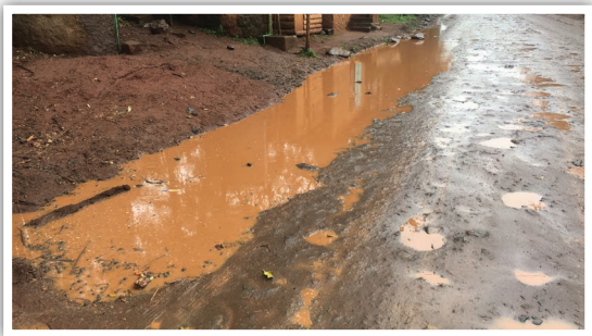
Eroded all area
