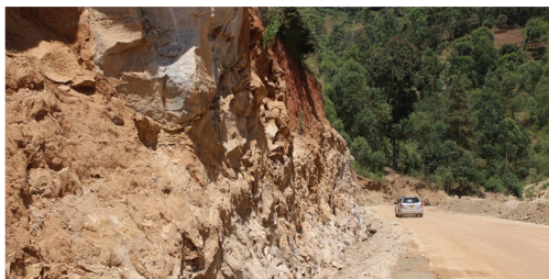
Slopes in cut is not stable
