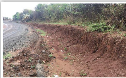
☒ Embankments slopes are deformed.
