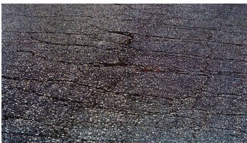
Typical transverse crack
