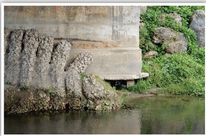
Erosion around bridge abutment
