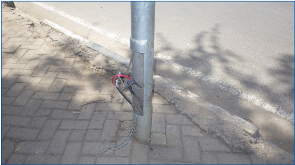
4. Lighting post without cover and reinforcement
