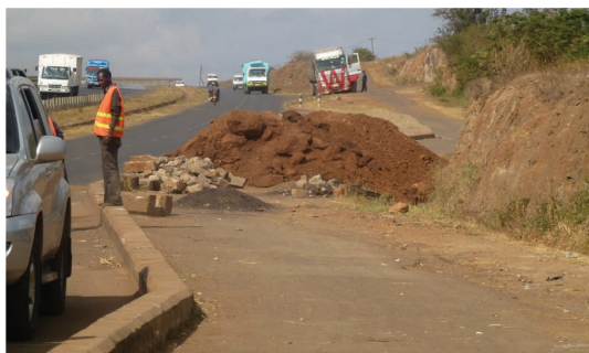
Absence of relevant warning signs
