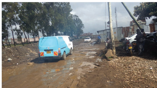
❌ Unacceptable level of gravel depth
