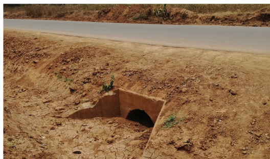
❌ Obstructed by soil deposit (case of pipe culvert)
