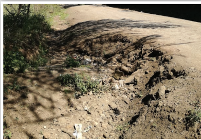
Damaged unpaved shoulders
