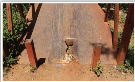
Damage of steel deck
