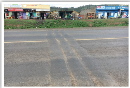
Absence of warning sign
