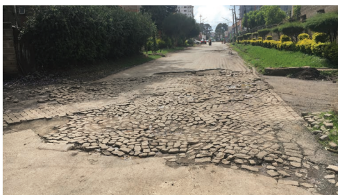
Obstructed by paving blocks
