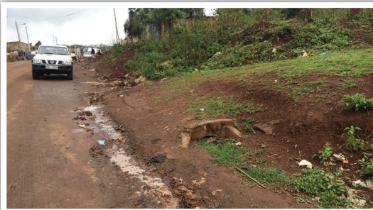
Blocked by weeds and soil
