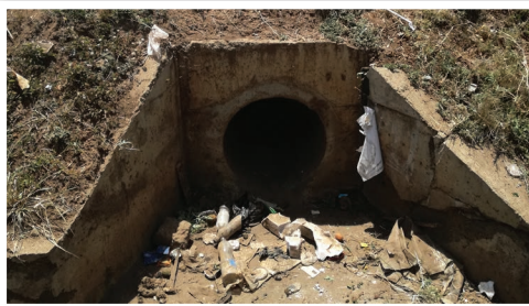
❌ Obstructed by debris
