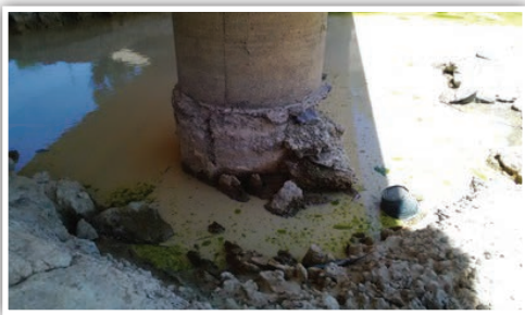
❌ A riverbed with debris and other obstructions
