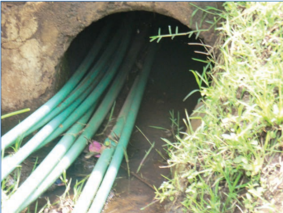
8. Culvert: Irregular occupation in culvert by utilities
