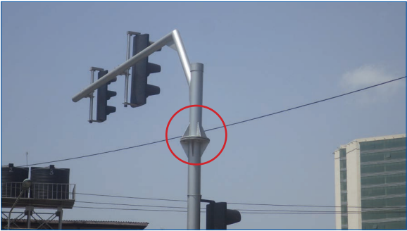
3. Incorrect jointing position flange
