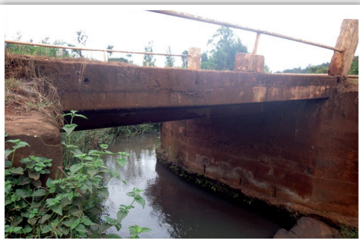
A damaged guard rail post
