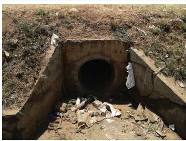
❌ Obstructed by debris
