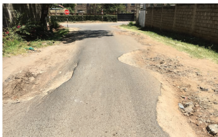
An unacceptable level of roughness
