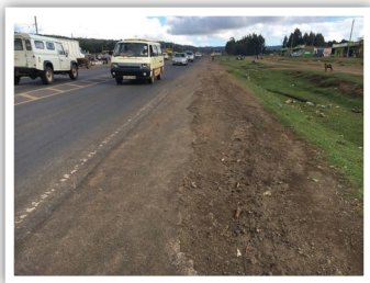
❌ Typical damaged paved shoulder
