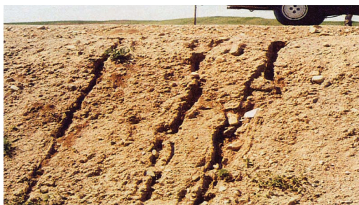
☒ Embankment slopes are deformed.
