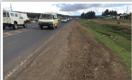
☒ A difference in height at edge of pavement
