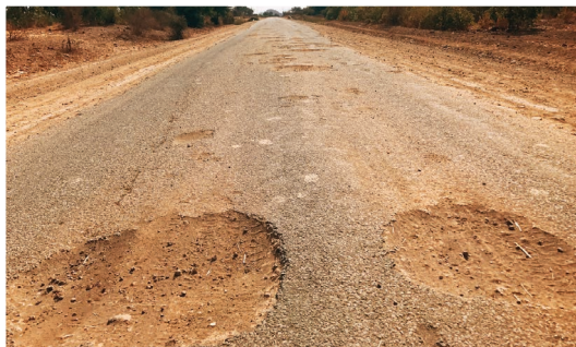
❌ Approximately 200 mm diameter pothole
