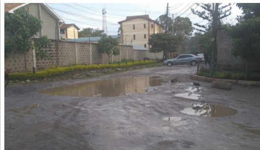
Approximately 200 mm diameter pothole
