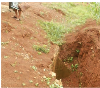
Obstructed by structural damage
